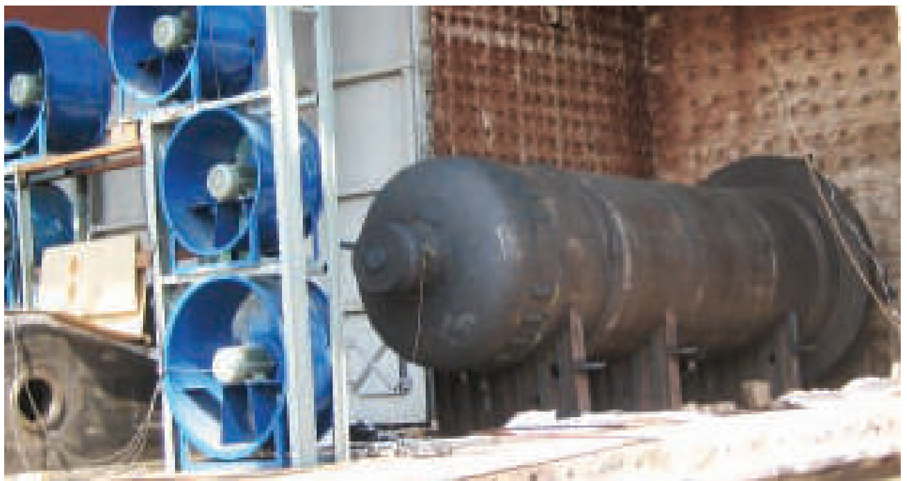
Forced Air Cooling SS claded Vessel
