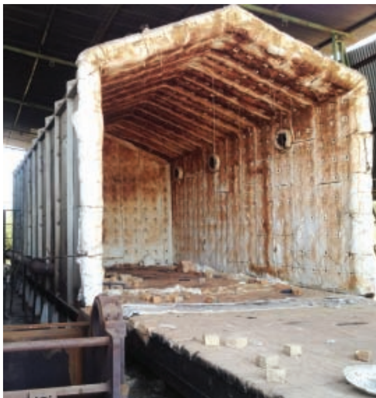
Ceramic Fibre Lining Bogie Furnace
