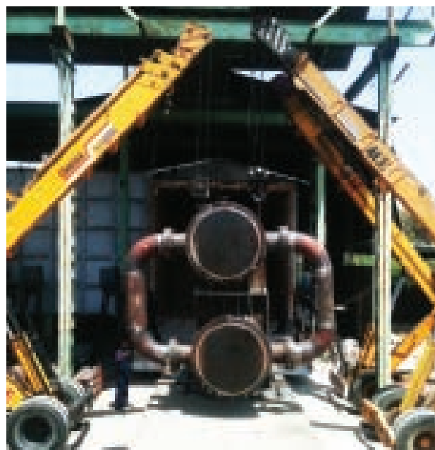
PWHT Heat Exchanger
